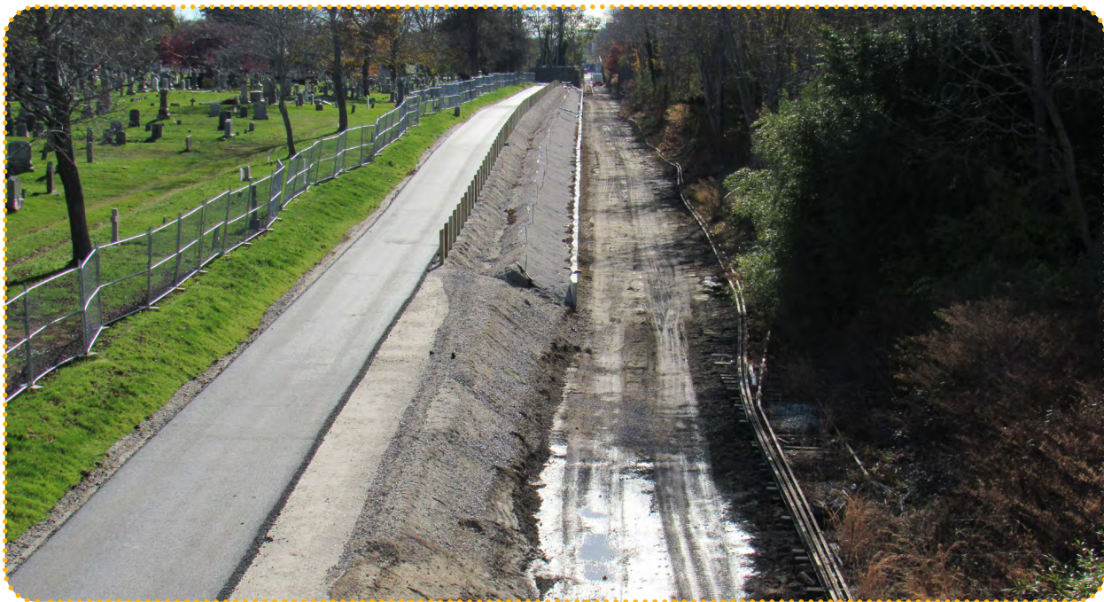
Trail under construction from Van Zandt Ave looking south to downtown Newport
